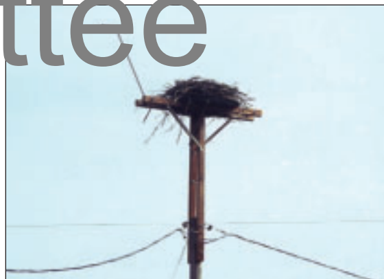
FIGURE 6.11: A nest platform built atop a pole using crossarms to extend the platform above the conductors. This design also includes an optional elevated perch to attract ospreys. The perch should be perpendicular to the prevailing wind.
