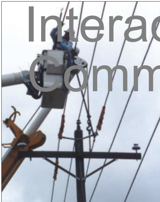
FIGURE 7.2: Reframing a crossarm to prevent avian electrocutions.
