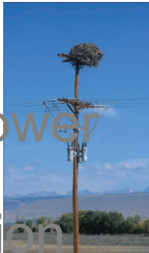
FIGURE 6.16: Osprey nest in Wyoming atop double dead-end pole. Nesting material that may drop onto the conductors or equipment poses fire, outage, and equipment damage risks.
